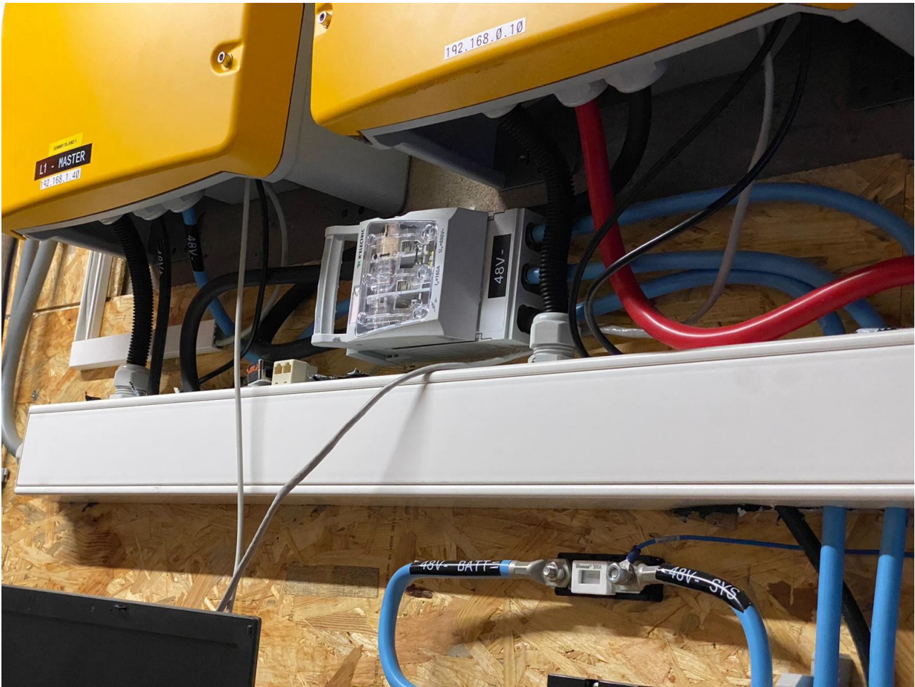
Use Blade manual breakers before inverters
